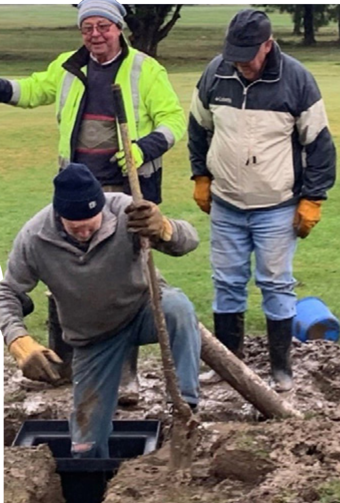
The pit for the drain behind the 8th green goes in during the break in lockdown restrictions.
